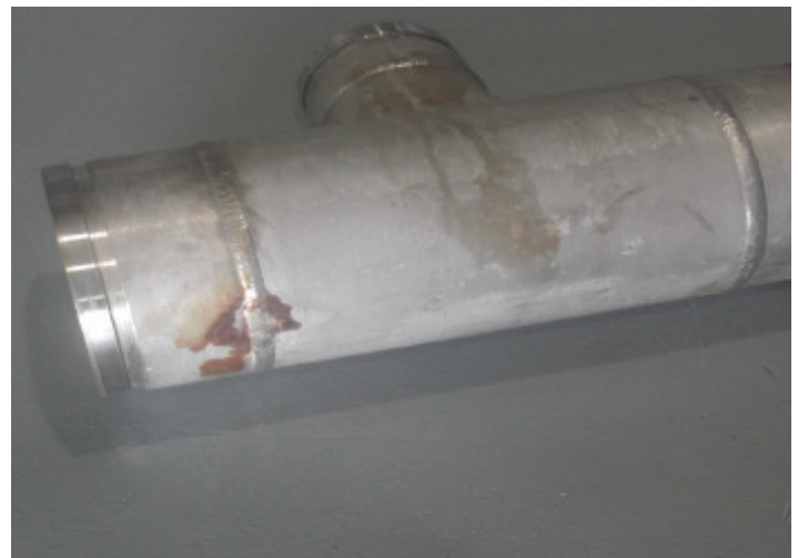
Figure 2 Corrosion and leakage of a superduplex weld due to precipitation of sigma phase in the HAZ.
