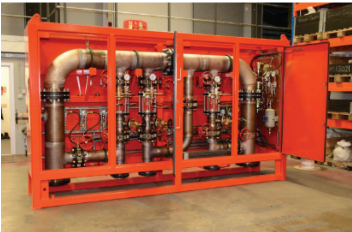
90/10 Copper-nickel deluge skid
