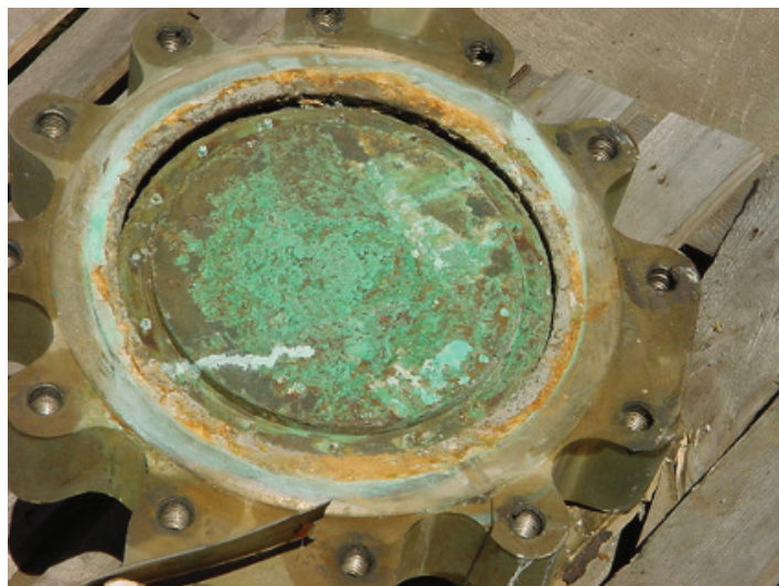
Figure 7 Badly corroded NAB valve from a superduplex stainless steel seawater line.
