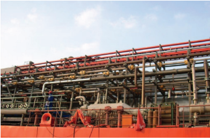
90/10 Copper-nickel piping on a tanker.
